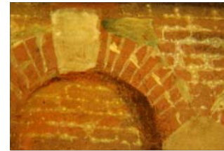
Closer detail showing the contrast between the bricks of the window arch (clearly painted with a brush) and the unusual texture of the brickwork section between the arches.
